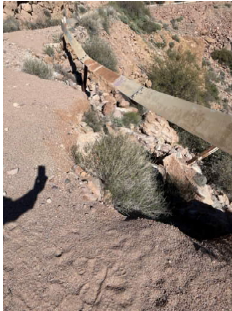
Photograph No. 5 – Erosion of roadbed and outboard slope at approximately MP 223 (looking north)
