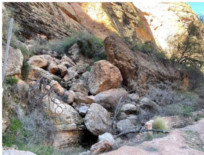
Photograph No. 4 – Rock debris flow near MP 222.4 (looking west)
