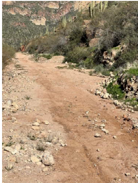
Photograph No. 8 – Series of debris flows adjacent to road at MP 223.9 (looking south)
