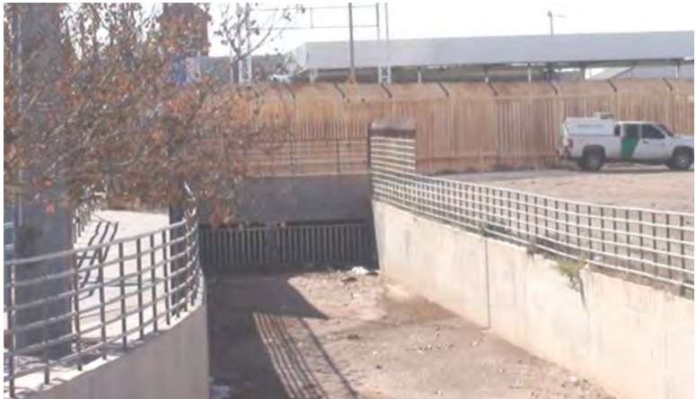
Concrete-Lined Drainage Channel on the West Side of Pan American Highways directly north of the Border
