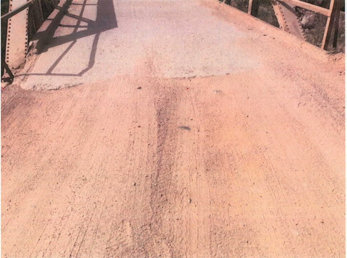
File Name : 00028-2018-08-30-Photo-F.jpg Description : Photo F – North Approach Condition
