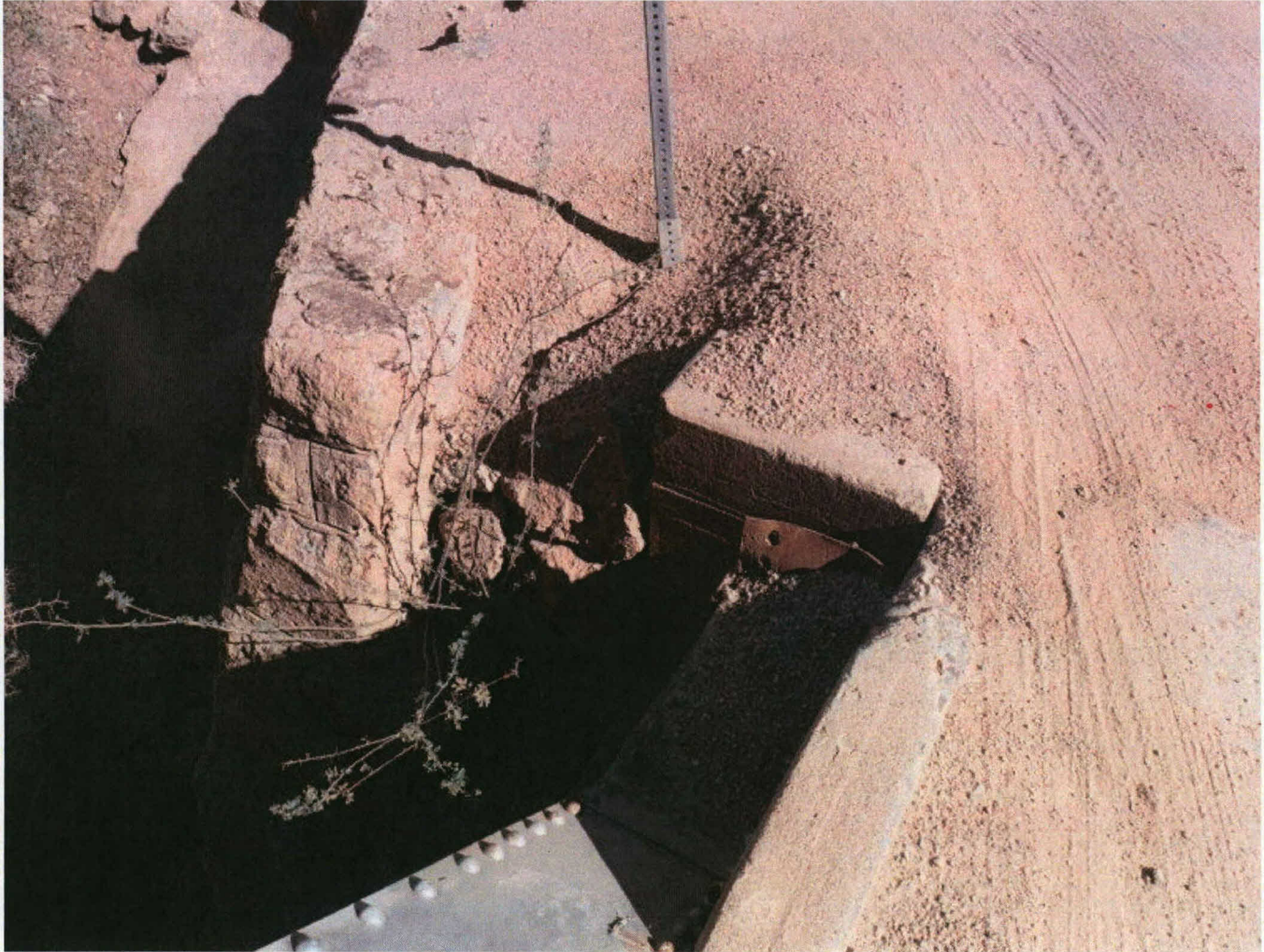
File Name : 00027-2018-09-08-Photo-G.jpg Description : Photo G. Northwest corner minor fill erosion
