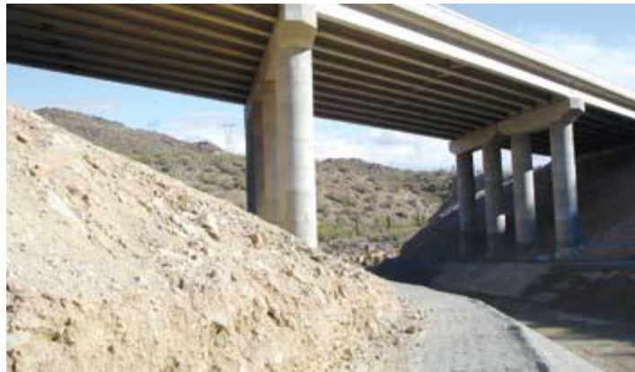
View of Cottonwood Canyon-Bridle Creek Bridge, designed to allow wildlife crossings Source: ADOT
