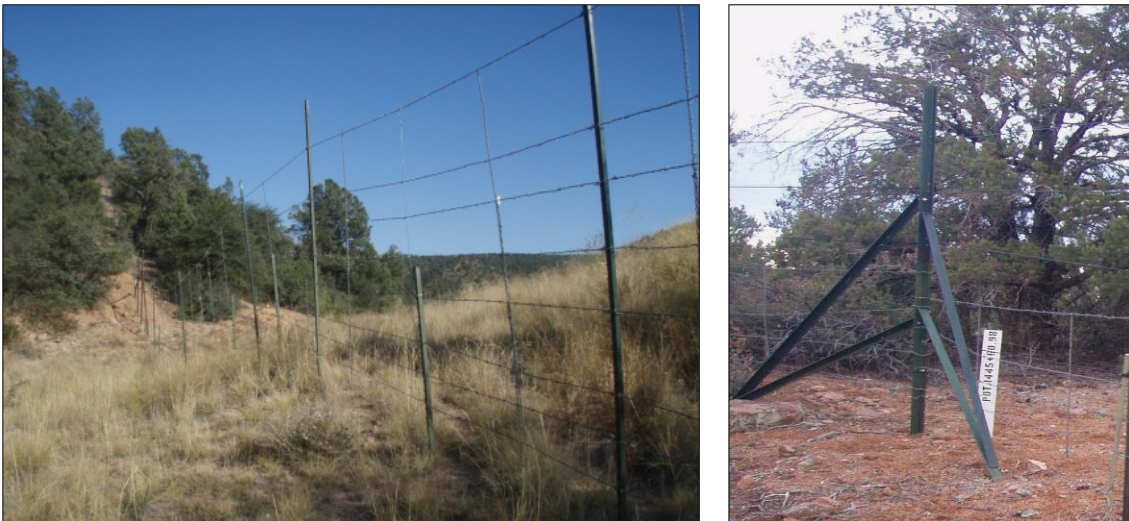
Figure 2. Application of retrofitted ROW fencing using 10-foot T-posts and barbed wire to extend the fence to 7.5–8 feet, with a metal in-line support posts for strength (left). Existing ROW fence corner braces were raised and supported with new angle braces bolted to the upright and bedded in concrete (right). Fencing retrofitted on State Route 260.
