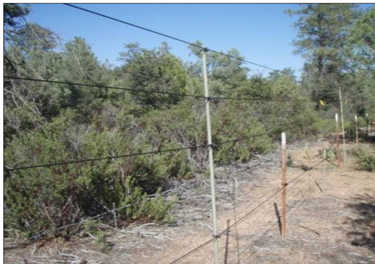
Figure 4. Application of modified ROW fence raised to 8 feet with ElectroBraid™ braided rope electric fence and fiberglass posts, with an electrified “kicker” mounted on the outside of ROW fence T-posts. Fencing retrofitted on State Route 260.
