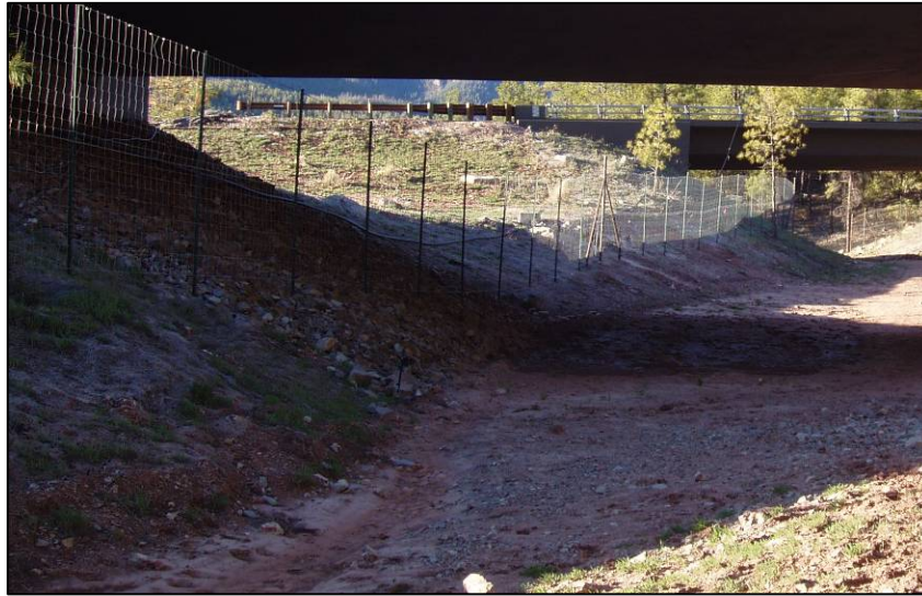
Figure 1. Standard 8-foot wildlife fence erected at a wildlife underpass along State Route 260. Note the woven wire, T-posts space 20 feet apart and metal support posts.
