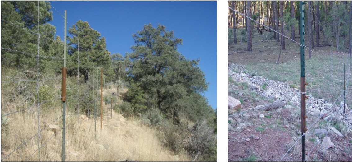
Figure 3. Application of retrofitted ROW fencing using T-post sleeve extensions and barbed wire to extend the fence to 7.5–8 feet, with a metal in-line support post for strength (left). Close-up of the T-post sleeve extending the existing T-post upward with bolts securing T-posts in place (right). Fencing retrofitted on State Route 260.
