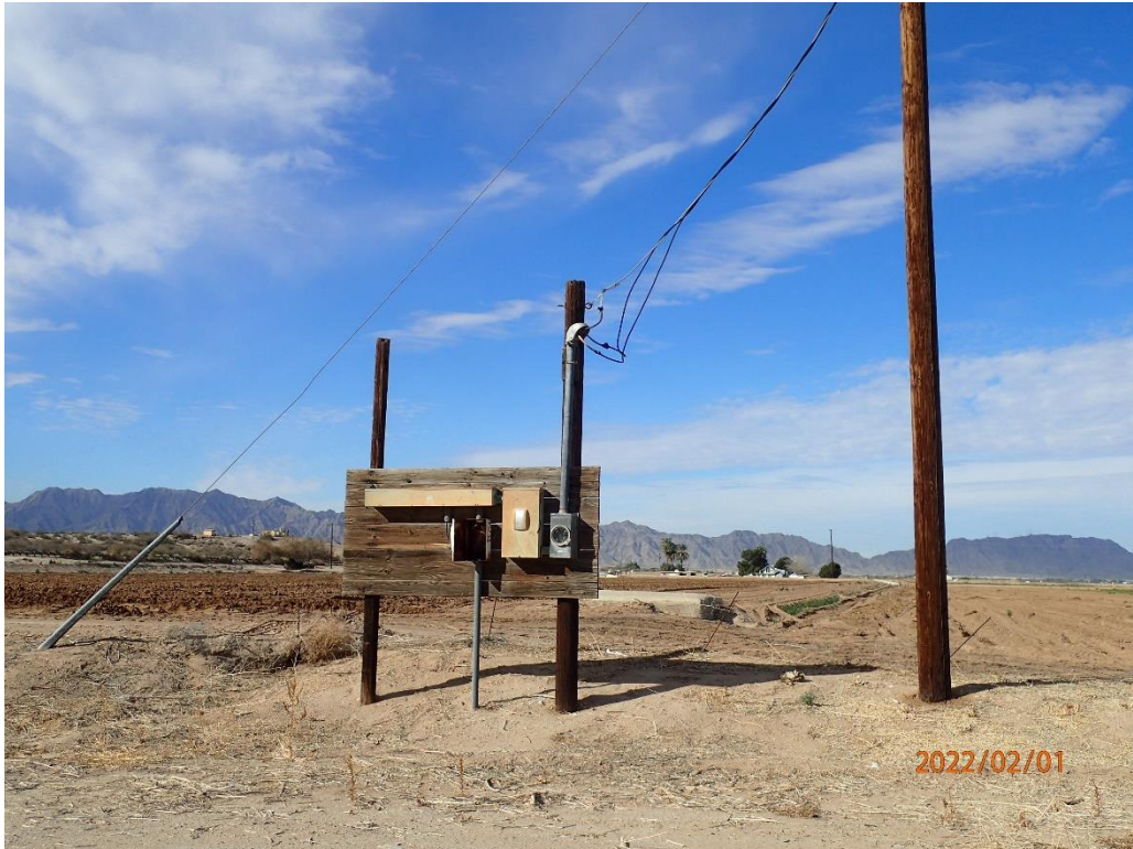
Electric service at west boundary. Meter removed.
