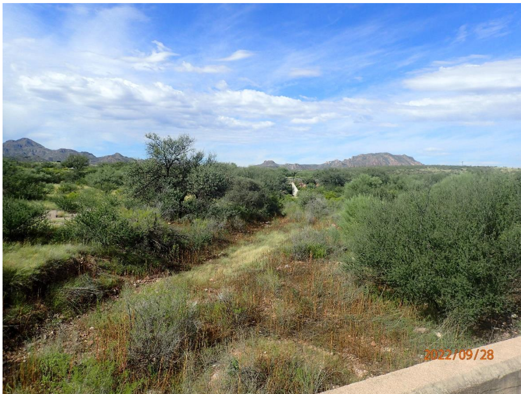
View west from old bridge to culvert under I-19 and Frontage Road.
