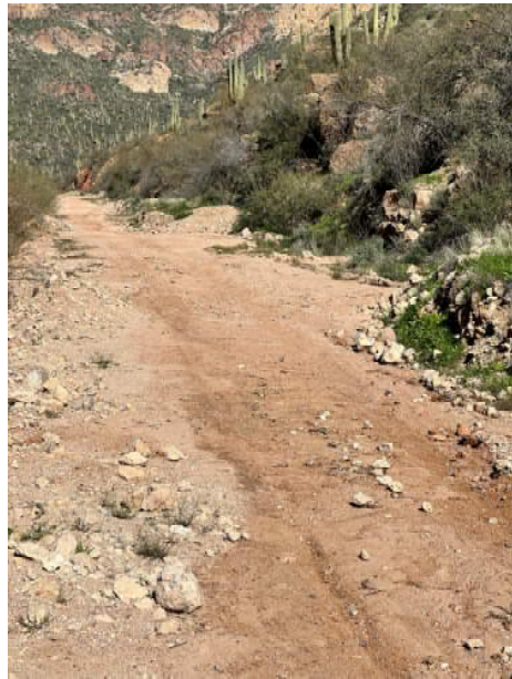
Photograph No. 8 – Series of debris flows adjacent to road at MP 223.9 (looking south)
