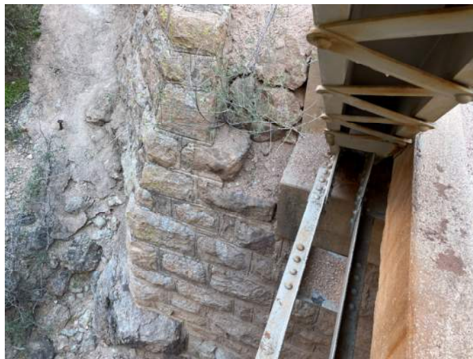
Photograph No. 6 – Northeast corner of Fish Creek Hill Bridge, East Abutment at MP 223.6 (looking east)
