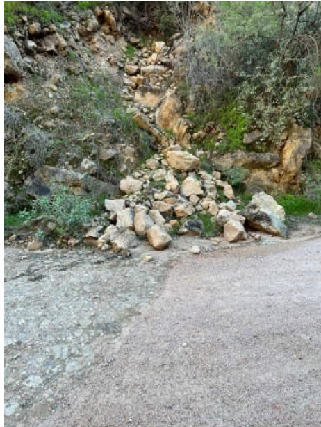
Photograph No. 7 – Rock debris within drainage at MP 223.9 (looking south)
