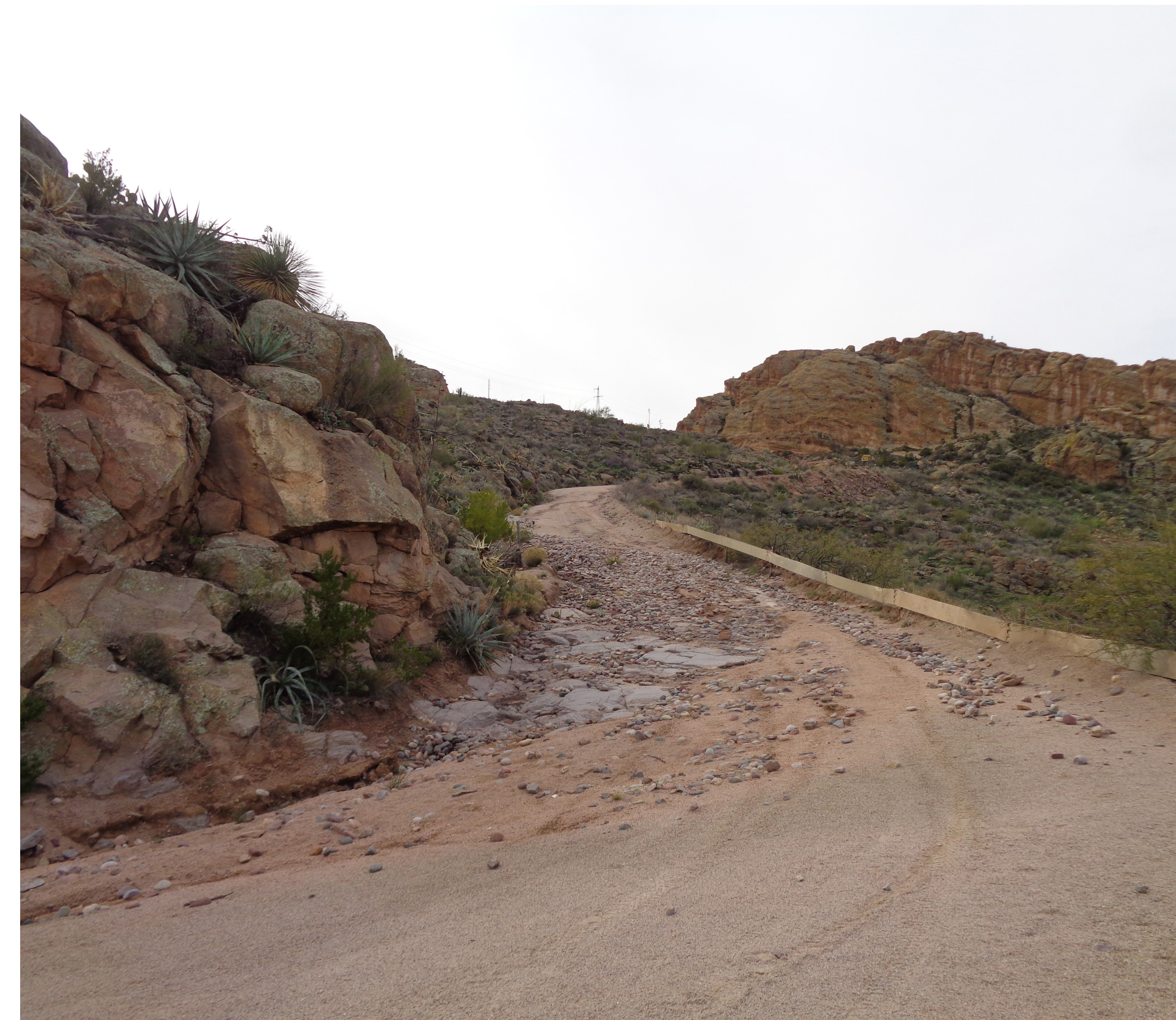
Narrow roadway, eroded surface
