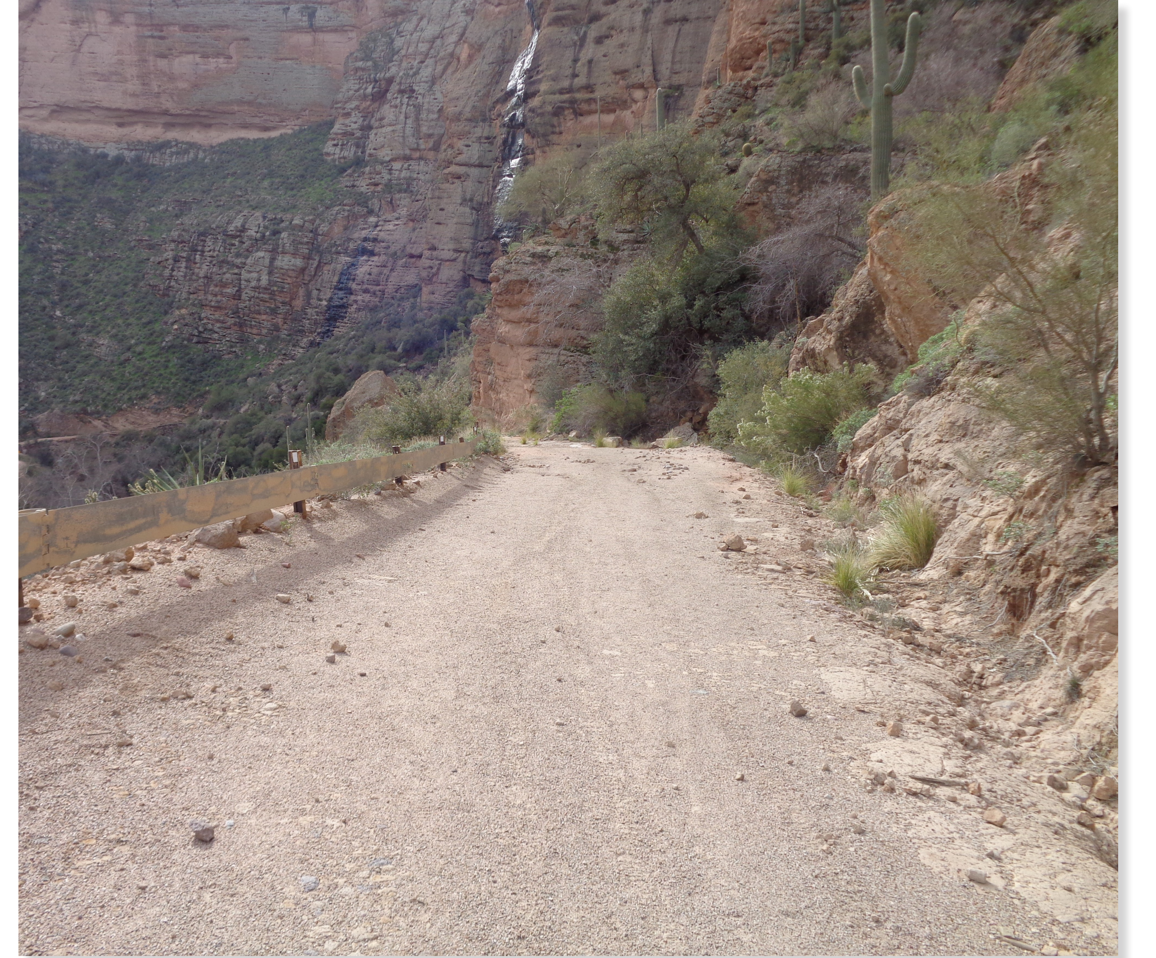
Guardrail is damaged and in poor condition
