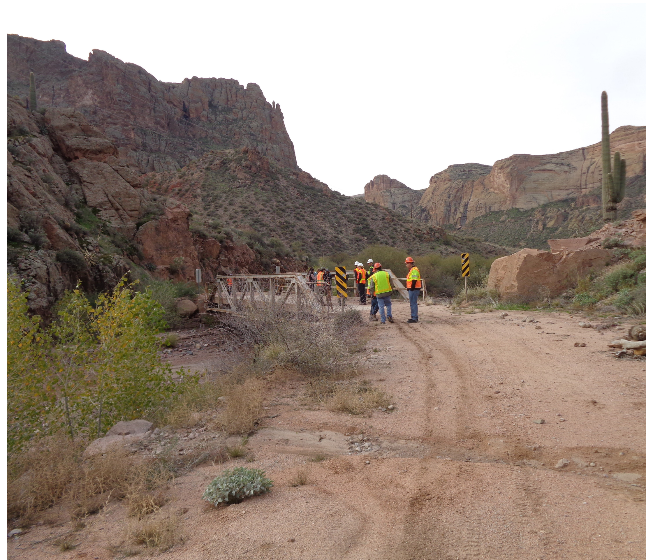
Bridge rehabilitation/repairs are needed
