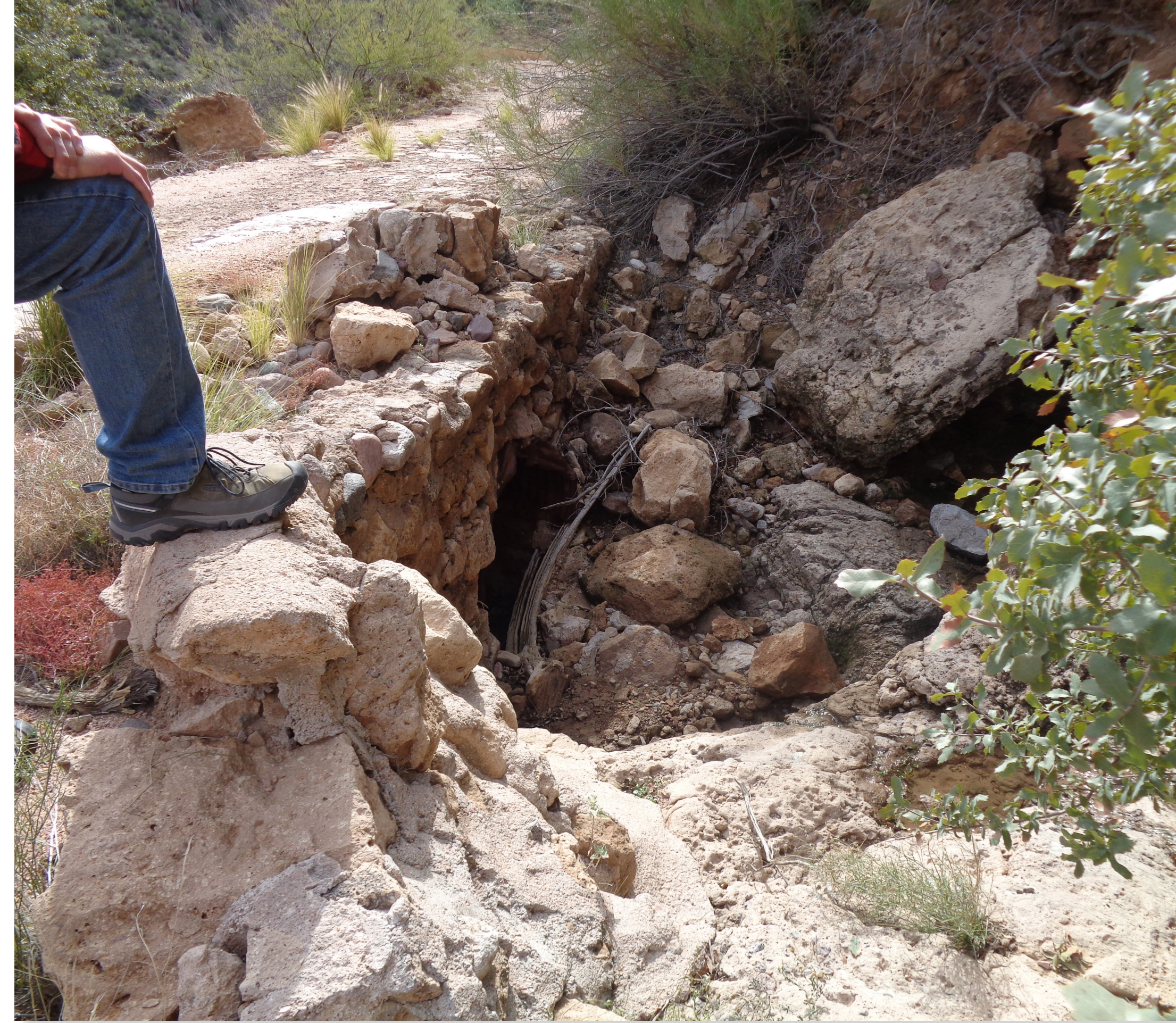
Drainage and erosion
