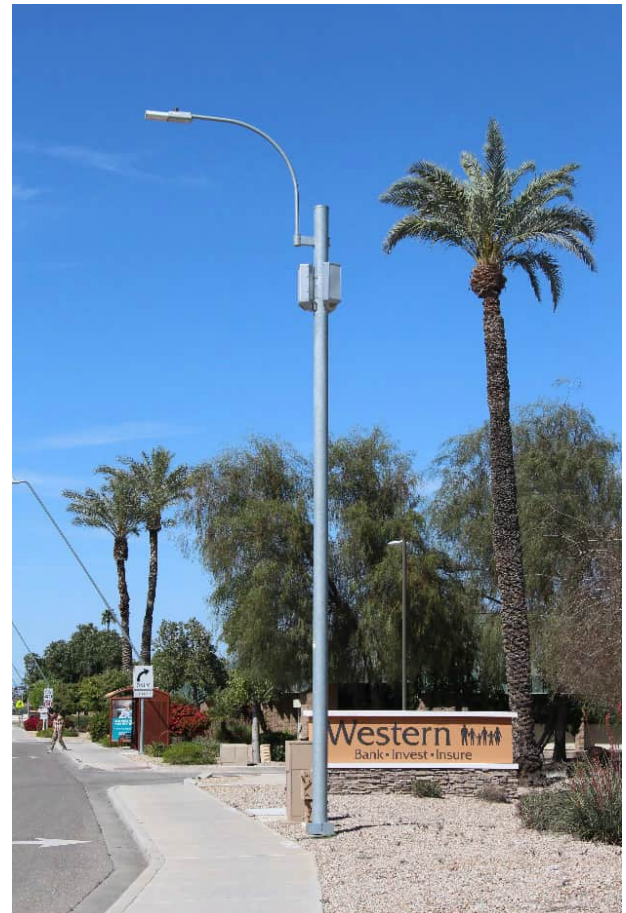
Figure 2: Example Collocation on a Roadway Luminaire Pole
