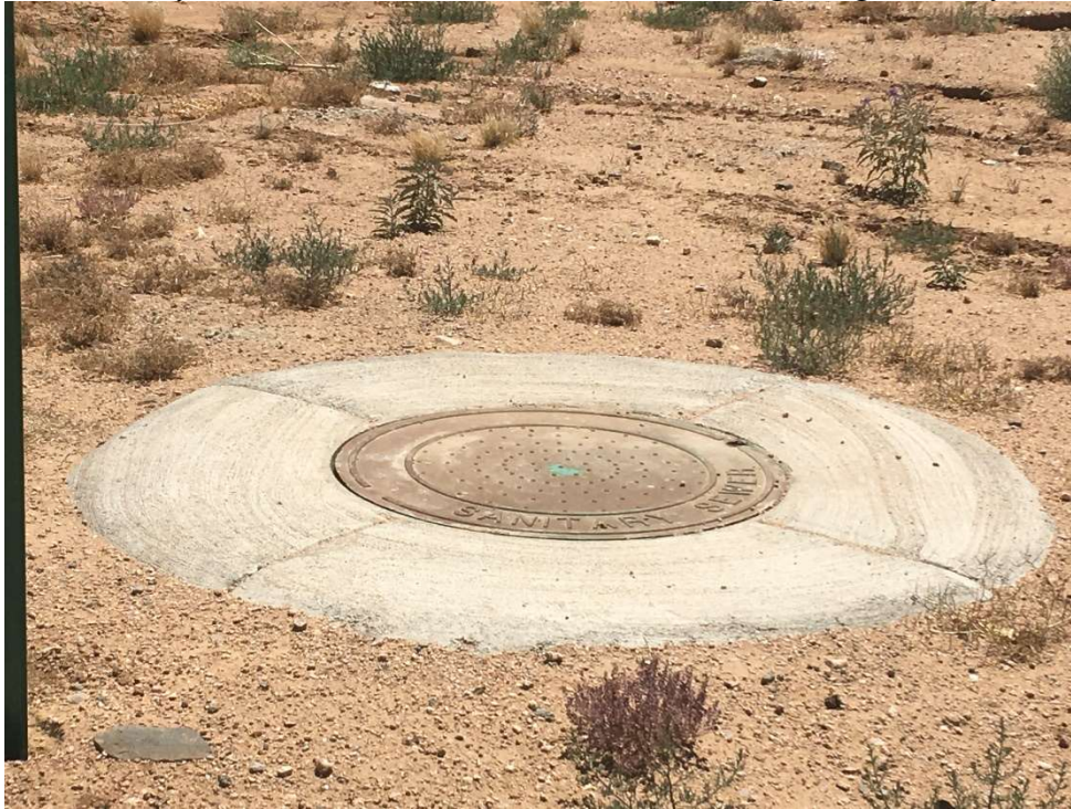
Sanitary Sewer Manhole Cover; inside Parcel C @ Diagonal Way
