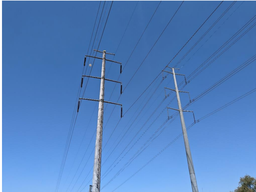
Electric poles on south portion of site (180007061)
