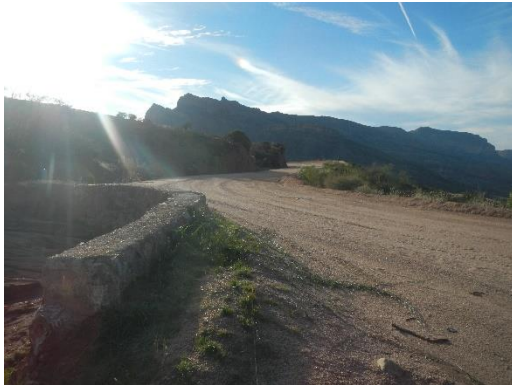
Figure 8. Slightly visible culvert headwalls following flood damage
