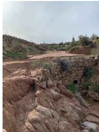
Figure 9. Highly visible culvert headwall following flood damage
