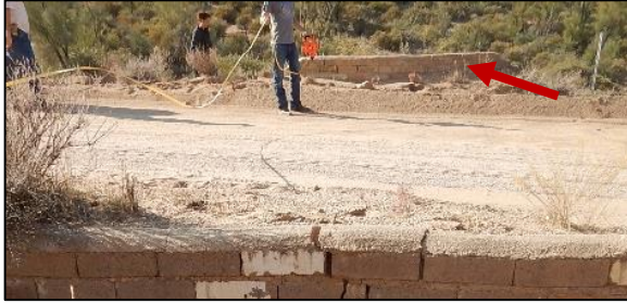
Figure 6. Slightly visible culvert headwalls prior to flood damage
