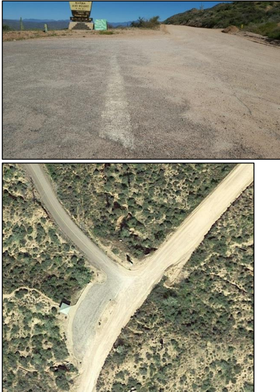
Figure 5. Road Surface at Intersection of Marina Access Road and Apache Trail
