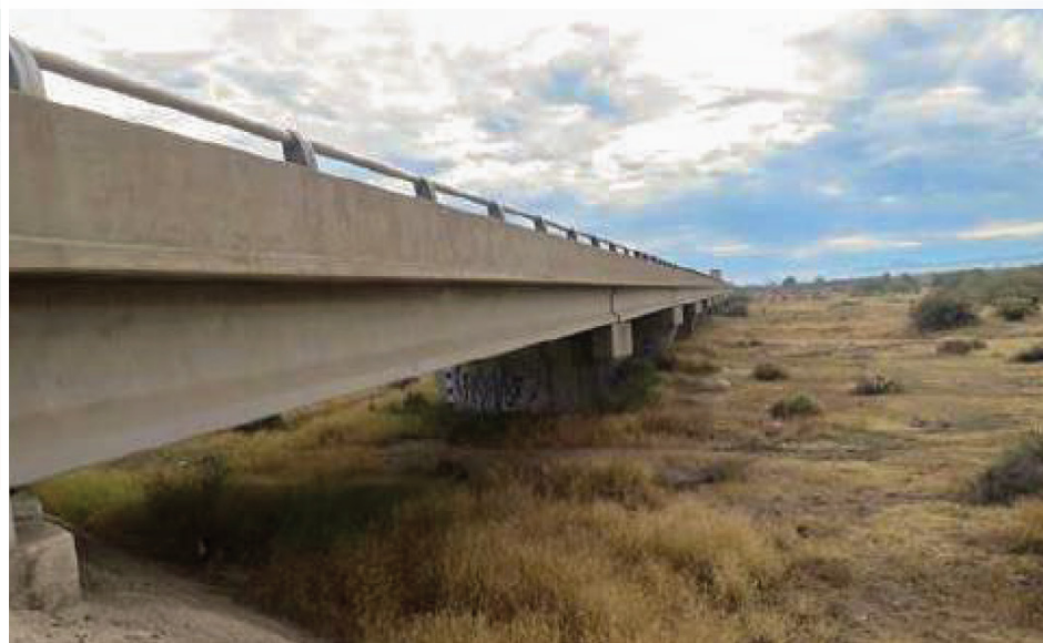
Below: This view of the Interstate 10 Gila River Bridge shows the low clearance under the structure.
