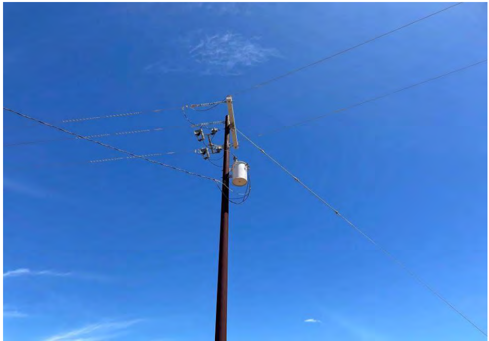
Photograph 15: View of a pole-mounted transformer at James Ranch Road.
