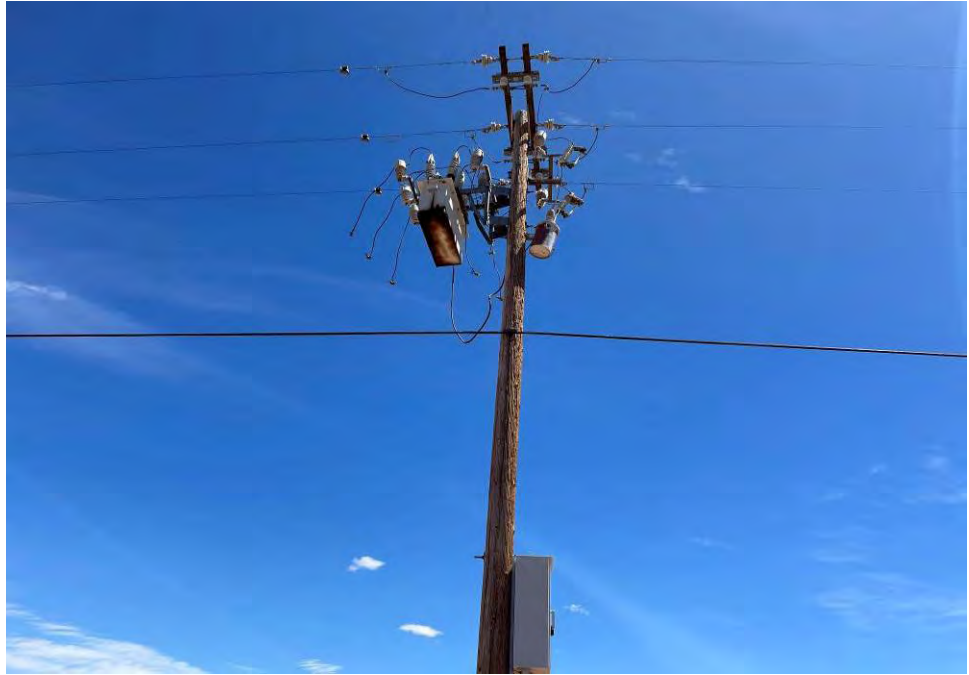
Photograph 9: View of a pole-mounted transformer on the northern portion of the Project Area north of State Route 80.
