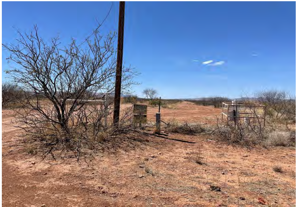
Photograph 25: View of high-pressure gas line cathodic protection on the eastern portion of the Project Area.
