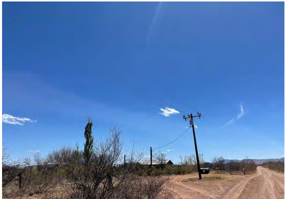
Photograph 12: View of a pole-mounted transformer at the residential property east of James Ranch Road.
