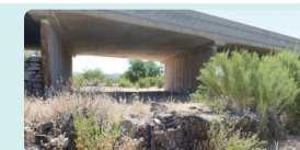
Removing the failing existing rail bank cut-off wall will result in long-term scour to reach equilibrium slope.
