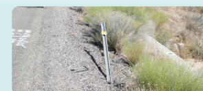
Existing culvert headwall with a damaged hazard marker within the clear zone.
