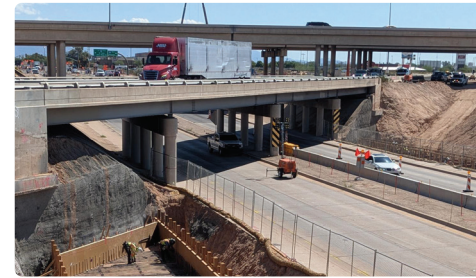
AECOM is currently providing CA services on the I-10/Kino Parkway DB (pictured). We understand the coordination and collaboration requirements of the DB delivery model.
