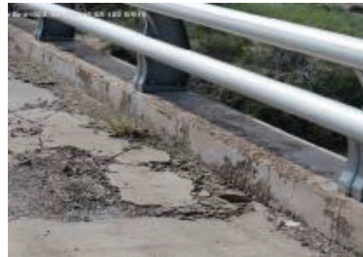
Figure 3-7 | Scaling on a Bridge Deck
