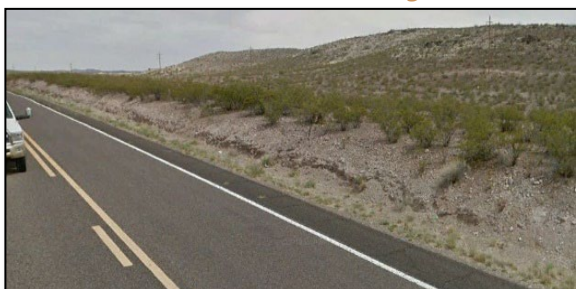
Minor: only one side of road with low slope
